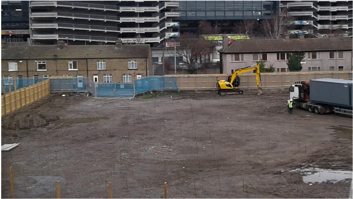
Demolition work on the main construction site at Croke Villas has been completed and construction work is set to begin.
